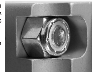
Fig 21 Bolt protrudes just beyond flush
